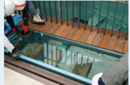
(4) Installation of glass flooring to allow pedestrians to see the restored railway tracks and sea surface
