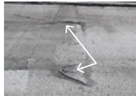
Reinforced bar exposure*
