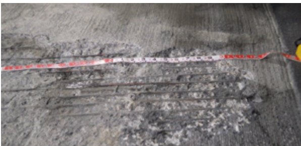
During pavement repair work, the underlying deck slab was found to be significantly damaged upon removal of the pavement, and the reinforcing bars were also corroded.
