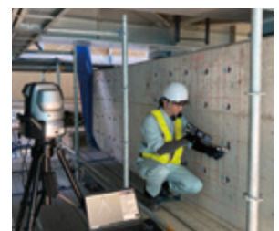
Status of measuring anchor bolt drilling positions using a 3D measuring instrument
