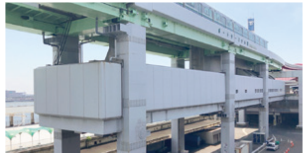
Railway construction project (completed seismic reinforcement of Kobe New Transit Port Island Line [PT Station and NK Station])
