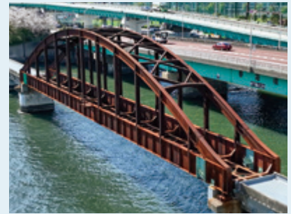
The former Harumi Railway Bridge prior to conversion work. The entire bridge coated in reddish-brown rust
