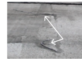
Reinforced bar exposure*
