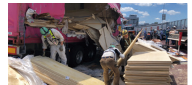
Cooperation in promptly reopening a road to traffic at an accident site (Tokyo)
