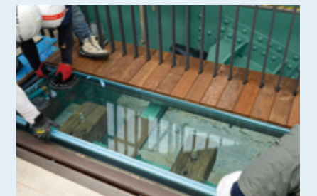
(4) Installation of glass flooring to allow pedestrians to see the restored railway tracks and sea surface
