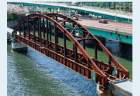
The former Harumi Railway Bridge prior to conversion work. The entire bridge coated in reddish-brown rust
