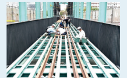
(2) After installation of the flooring base, the original rails from the time of operation were restored.
