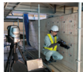
Status of measuring anchor bolt drilling positions using a 3D measuring instrument
