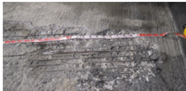
During pavement repair work, the underlying deck slab was found to be significantly damaged upon removal of the pavement, and the reinforcing bars were also corroded.
