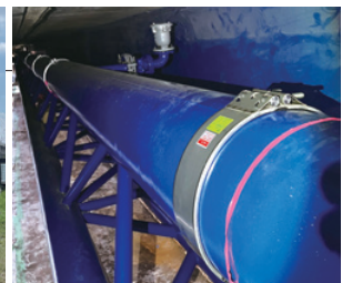
A utility water pipe bridge using SHO-BOND MATERIAL couplings
