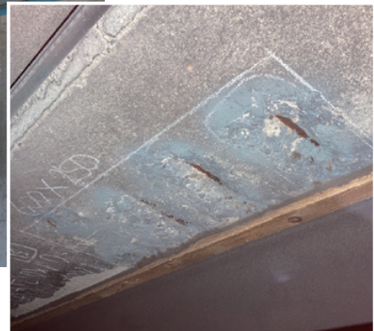
A section of spalling concrete
