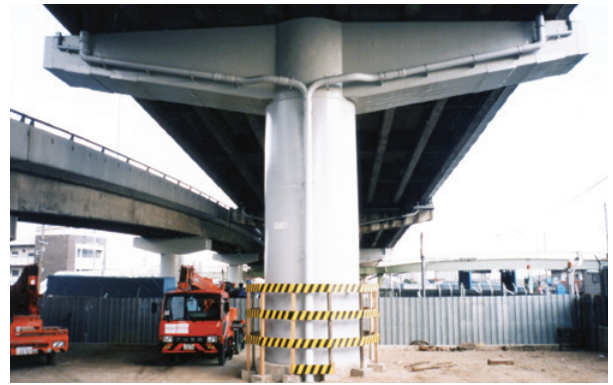
Piers of the expressway bridges reinforced shortly before the 1995 Kobe earthquake were not damaged by the powerful tremors
