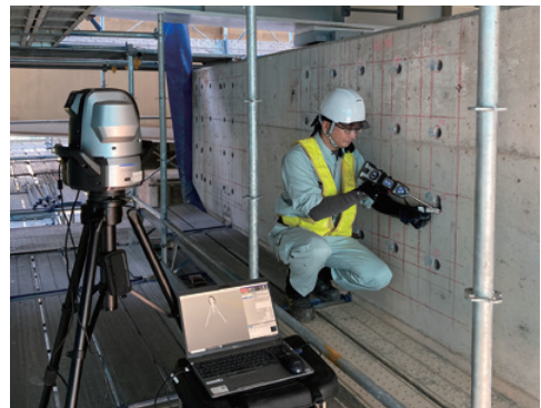
The status of measuring anchor bolt drilling positions using a 3D measuring instrument
