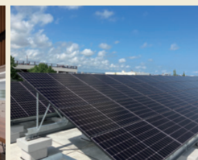
Rooftop solar panels
