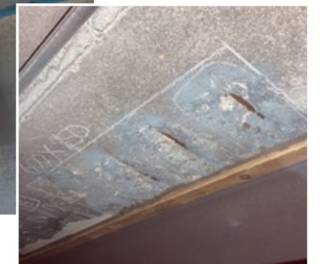
A section of spalling concrete
