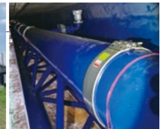
A utility water pipe bridge using SHO-BOND MATERIAL couplings
