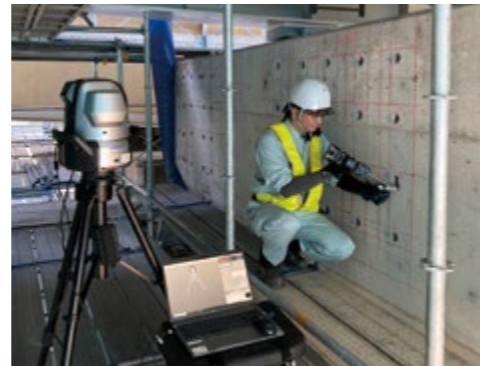
The status of measuring anchor bolt drilling positions using a 3D measuring instrument
