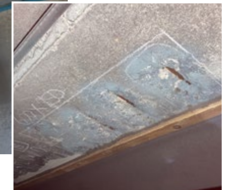
A section of spalling concrete
