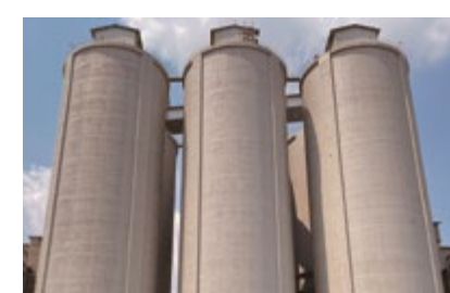
Silo Repair of wall surface degradation
