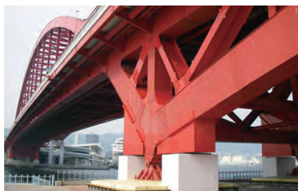
2011 SHO-BOND's work at the Kobe Ohashi Bridge received a Technology Award from the Japan Society of Civil Engineers Kansai Branch
