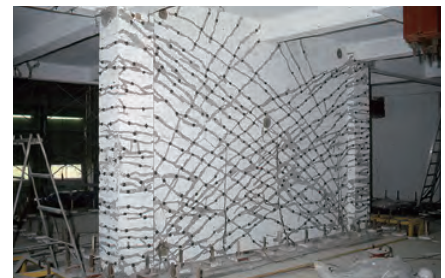
1981 The SHO-BOND BICS (Balloon Injection for Concrete Structures) Method for repairing cracks in concrete was used at the Japan-U.S. large earthquake resistance experiment at the Building Research Institute of the Ministry of Construction.
