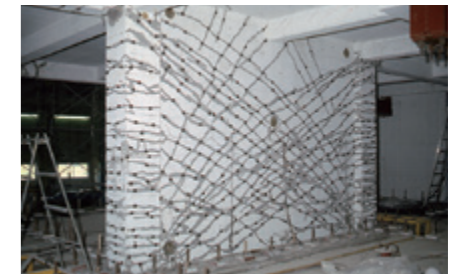
1981 The SHO-BOND BICS (Balloon Injection for Concrete Structures) Method for repairing cracks in concrete was used at the Japan-U.S. large earthquake resistance experiment at the Building Research Institute of the Ministry of Construction.
